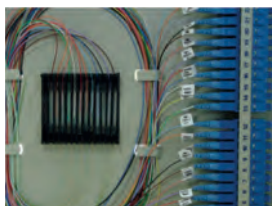
Accommodation of pigtails and splicin
